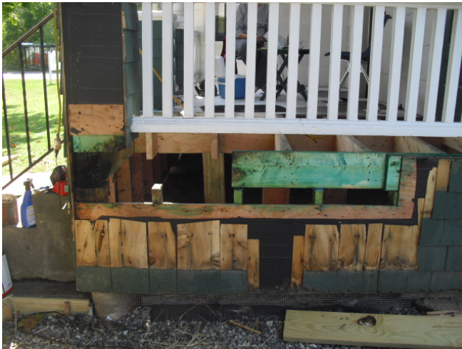
Rotting framework on the back porch.
